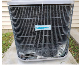
Deterioration due to pet urine
