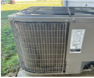
Accumulated dirt on A/C Unit
